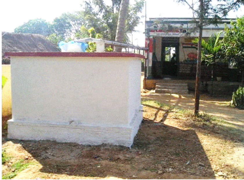
Fig: A storage tank on a platform painted white
